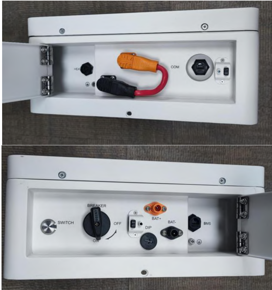
Communication connection of Main control unit
